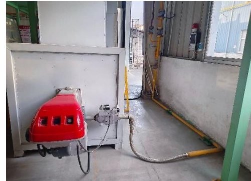
Natural Gas Heating
